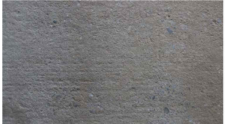
▲ A bare concrete floor where only screeding was done.
